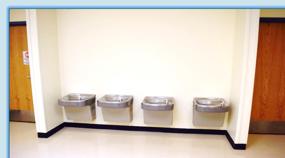
Cuba Elementary School water fountains
