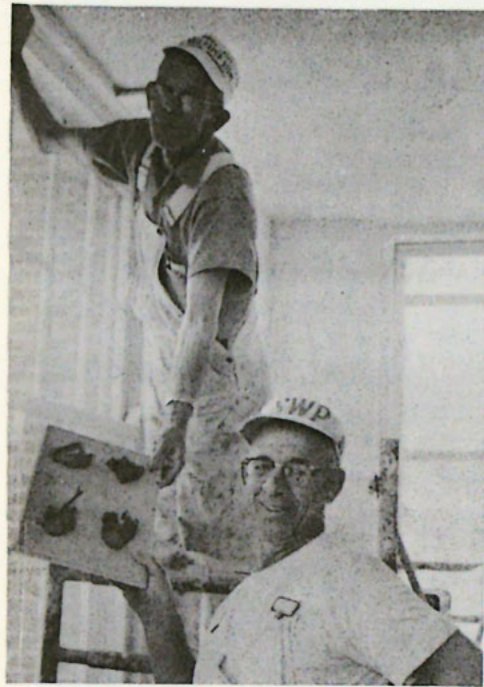
Refinishing the ceiling of the main dining room with acoustical tile was the job of painters Carl Dinndorf, top of picture, and Tony Malikowski.
