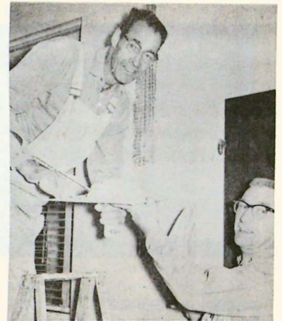
Plastering the walls are Gus Deppa, left, and Nick Binsfeld of the hospital maintenance crew.
