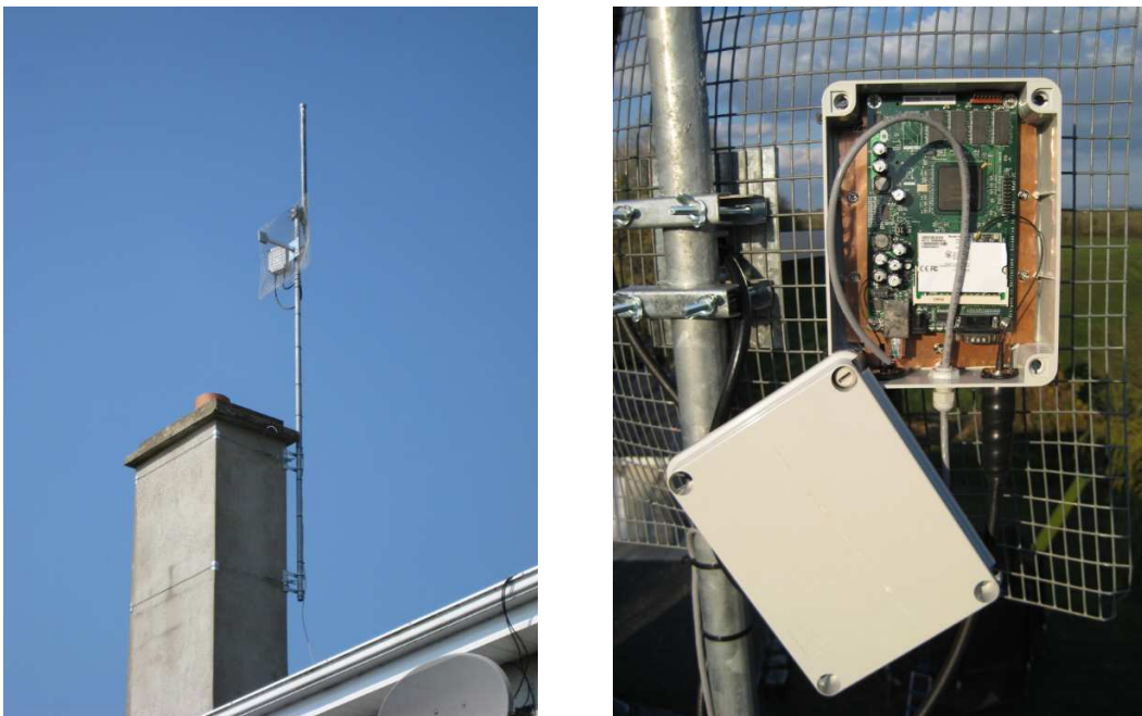
Figure 6 Live installation example
