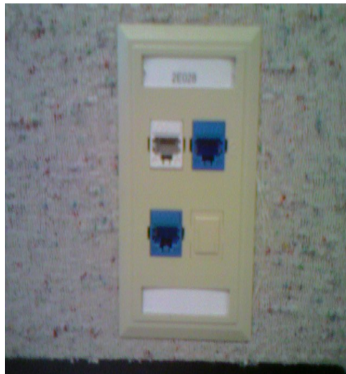
Cube Wall Data Ports
