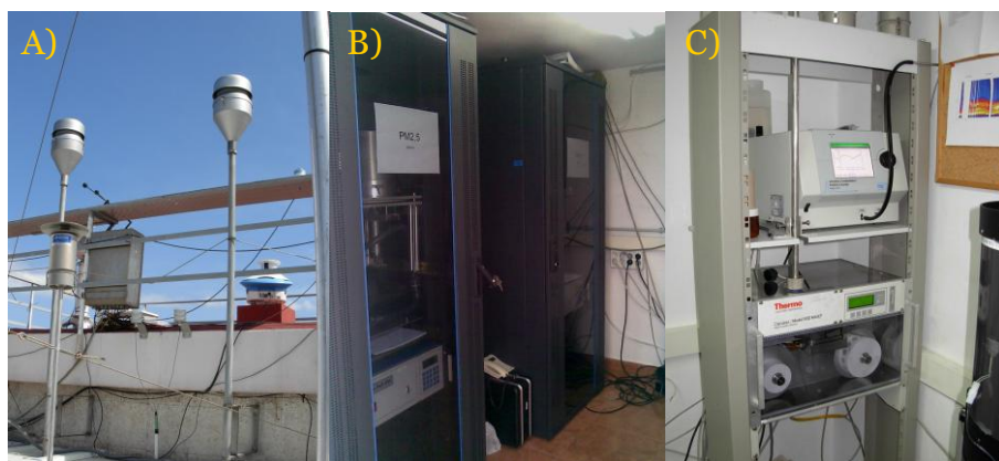
Figure 2.25 Inlets (A) and indoor view (B-D) of SCO
