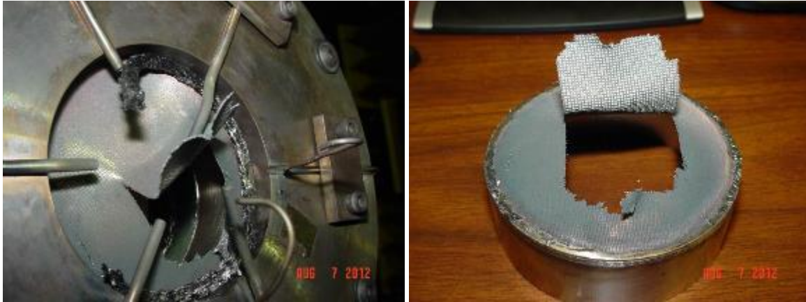
Figure 38 Second Screen Flow Conditioner Failure. (12)
