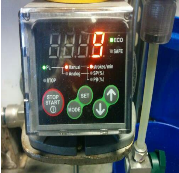
Figure 33 Conducting pump trial settings
