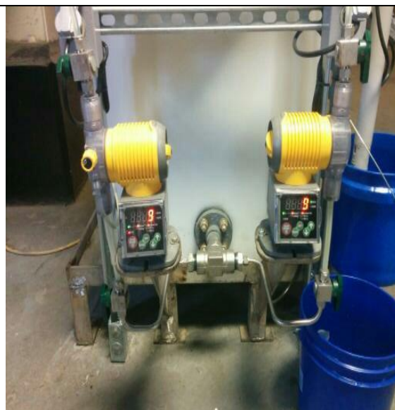
Figure 28 Chemical System Installation at Hampton Plant
