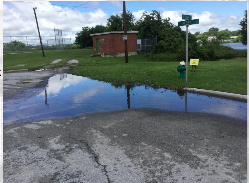
Tidal Flooding and Runoff near a Sewer Pump Station
