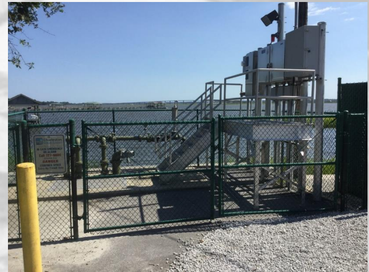
Pump infrastructure...and elevation
