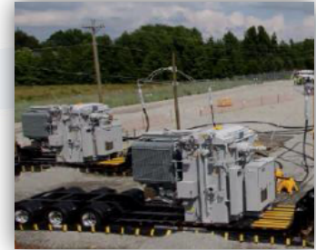
Transmission Mobile Transformers
