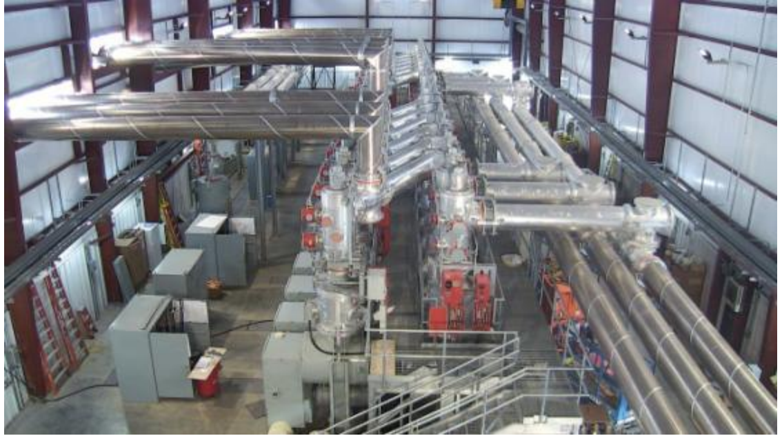
Gas Insulated Switchgear mounted indoors
