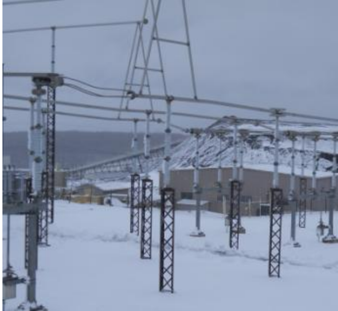
Use of Resistive Glaze Insulators Or Stepped Shed Designs
