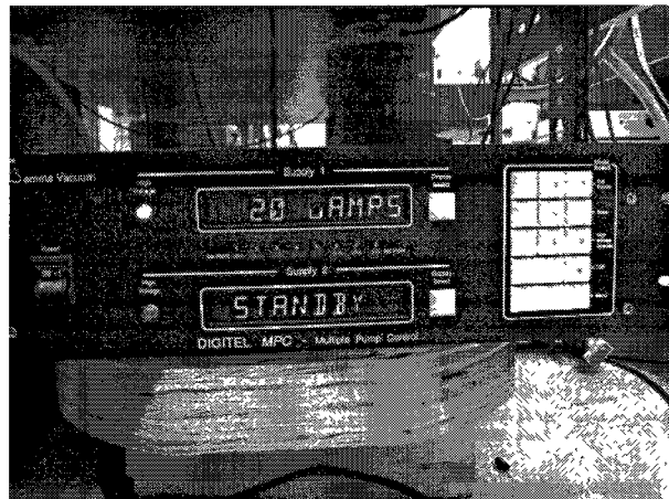
FIG. B-3 The ion pump power supply
