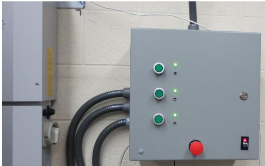
Figure 3.14: PV load switching enclosure.
