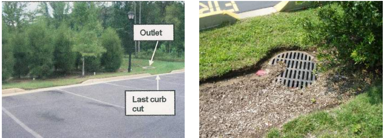
Figure 9.11. Examples of Short-Circuiting at Bioretention Facilities
