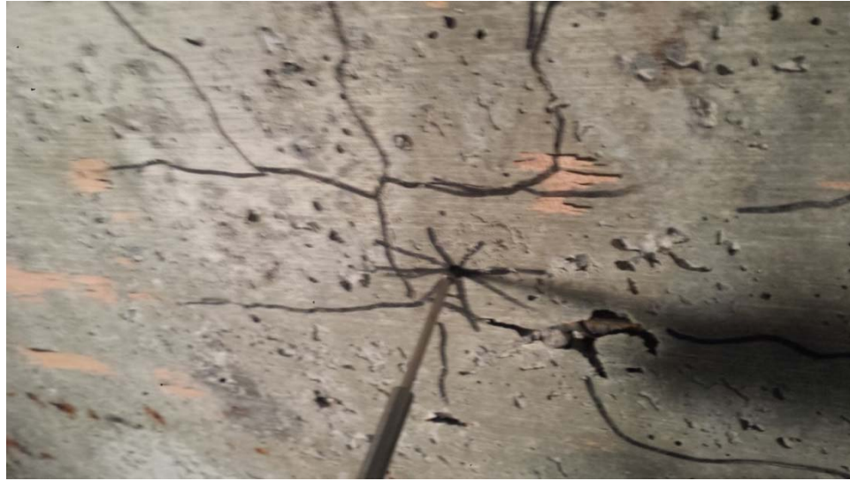
Figure 107. Cracks at the bottom surface of slab in SL01
