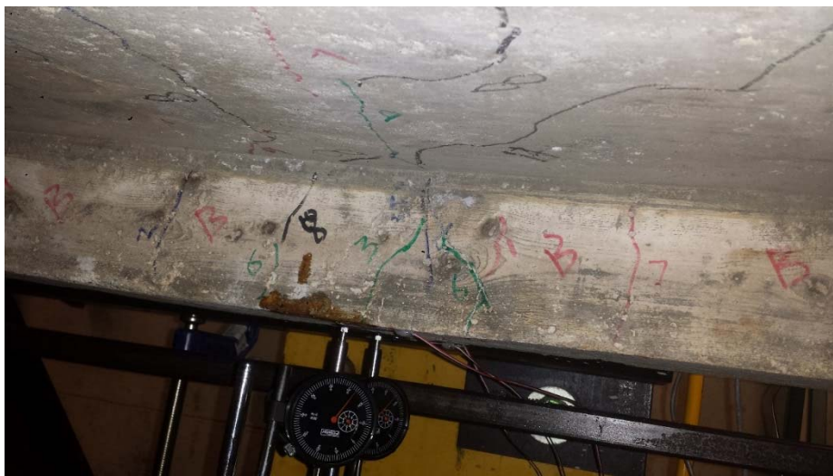
Figure 118. Final crack pattern of SMB in SL03
