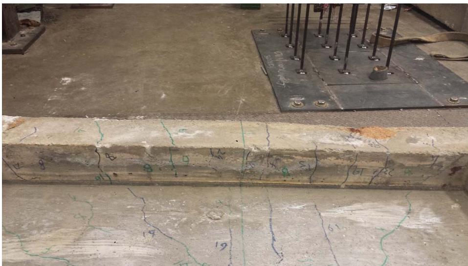
Figure 113. Final cracking pattern in typical spandrel member of SL02
