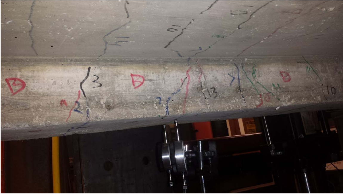
Figure 119. Final crack pattern of SMD in SL03
