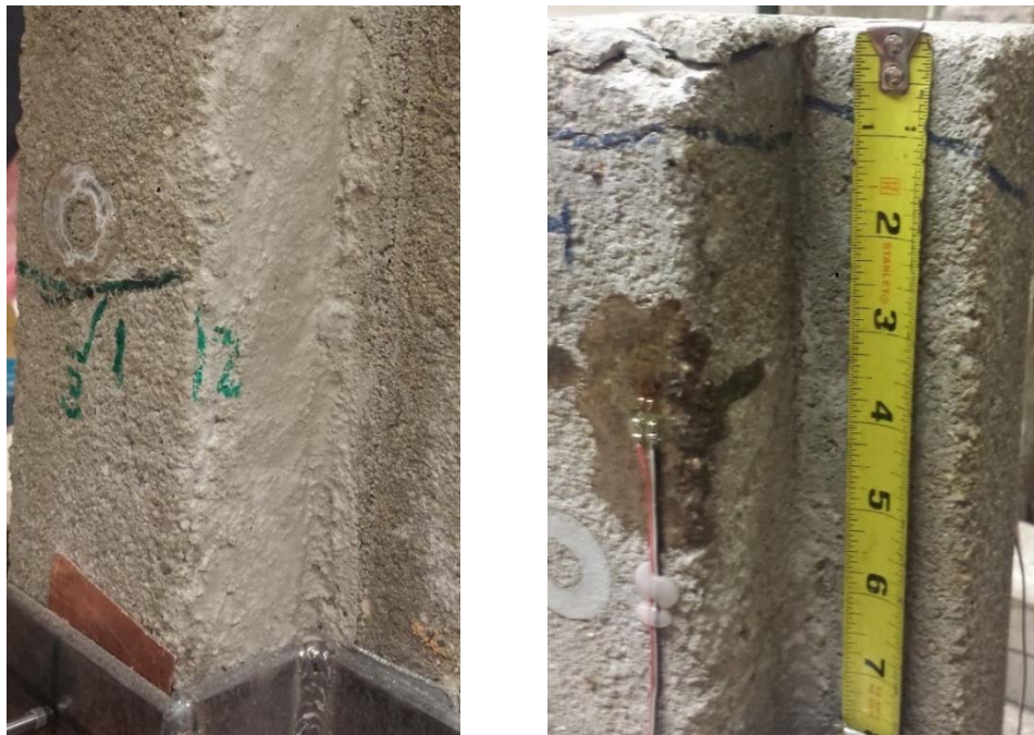
Figure 101. Final crack pattern for SM18
