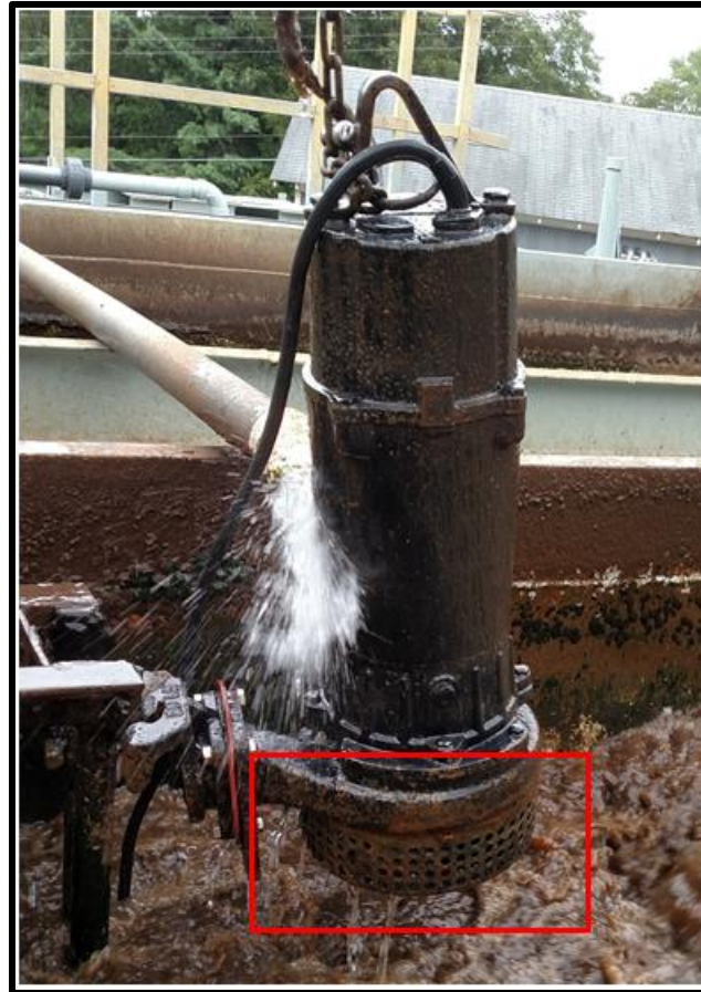
Figure 8. Ebara submersible feed pump for the external selector showing the suction screen at the UB WWTP.
