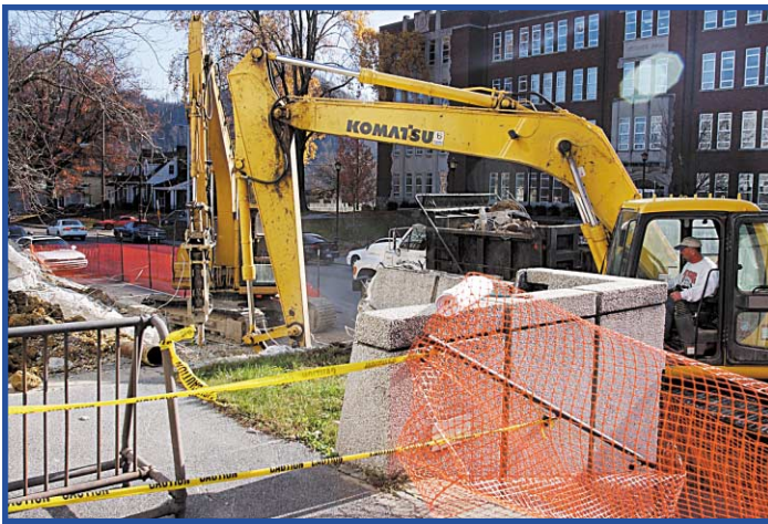
Work progresses on the ADUC renovation project, and traffic has been re-routed through the campus.
