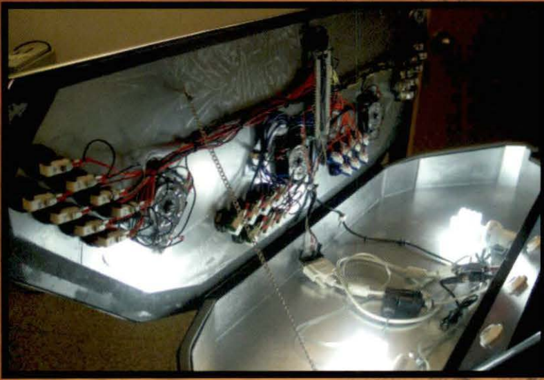
Wiring system for the keypad
