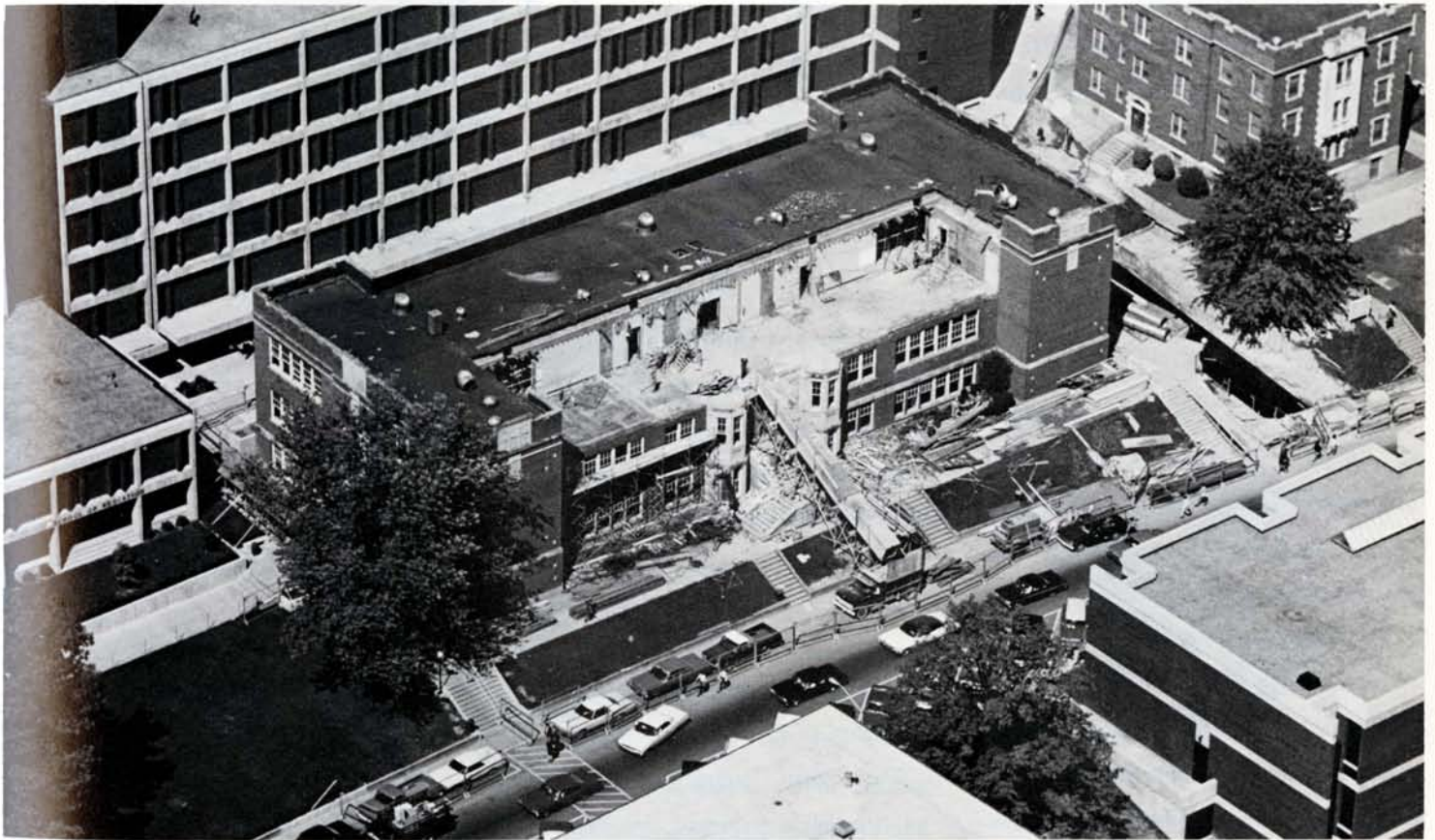
TRANSITION — Typical construction scene during the Doran years is this aerial view of the renovation of Rader Hall, once the administration building. At right is old
