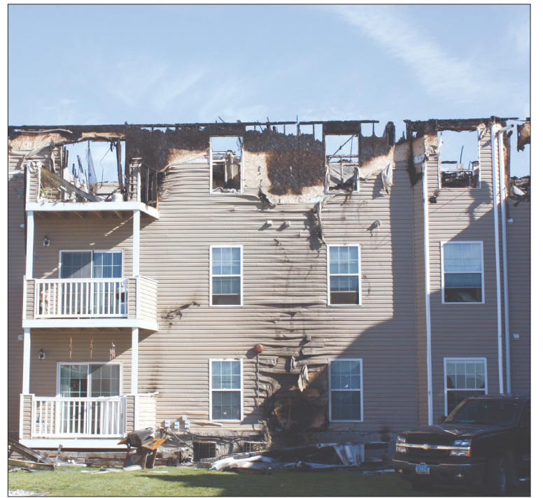
The fire at the Galleria apartments in south Fargo left many without a place to stay for days. Robert Jacobson • The Advocate
