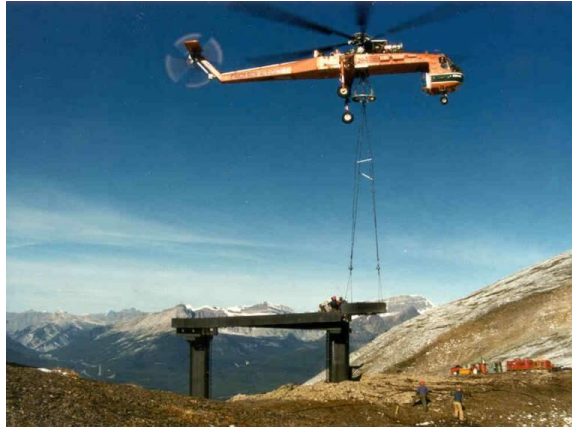
Fig. 1.3 A ski resort being assembled in Canada (Reprinted with permission from Judy Shellabarger Gosnell)
