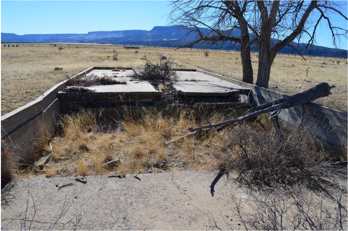
Figure 39. German Officer's Theater, note the hole between the slanted floor and raised flat stage area.
