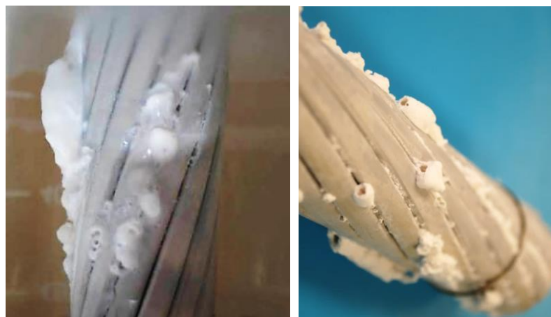
Figure 24: Formation of \text{Al(OH)}_3 on the aluminum strands in a transmission line conductor sample. Left) Sample that is still wet; Right) Dried sample.
