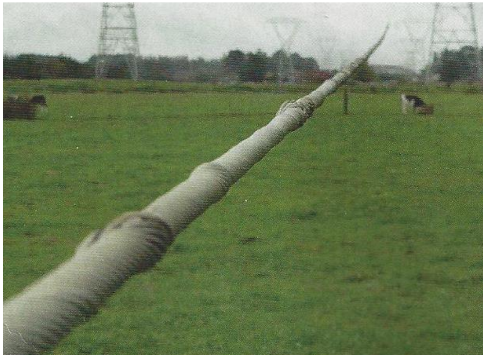
Figure 7: Bulging of ACSR conductor due to build-up of corrosion products. From (Renton 2013)
