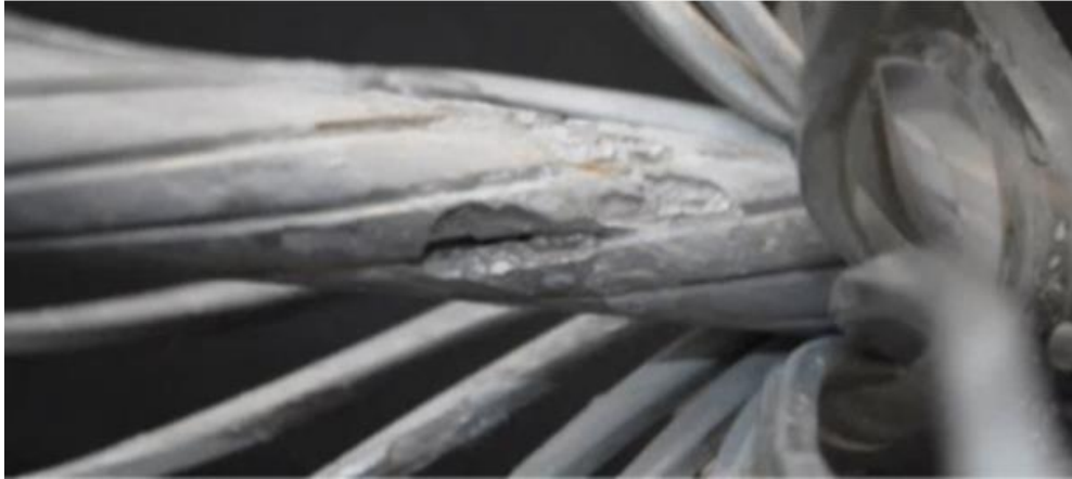
Figure 27: Typical pitting corrosion of aluminum. The strands of an ACCC conductor after 3 months submersion in 85°C, 3 mass % NaCl aqueous solution.
