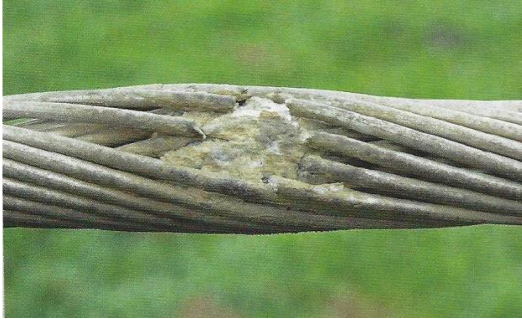
Figure 8: Severe corrosion damage on ACSR conductor after 35 years in service in New Zealand. From (Renton 2013)
