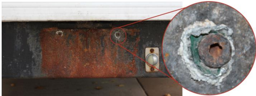
Figure 16: Trailer license plate lost due to galvanic corrosion between the steel screws and the Al plate. The corrosion was caused by exposure to NaCl, MgCl 2 and other salts during several trips to the Bonneville Salt Flats, Utah. The original green paint from the license plate can still be seen on top of the aluminum corrosion products.
