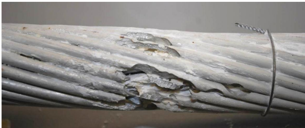
Figure 66: Severe localized corrosion on the ACSS sample after Test A.
