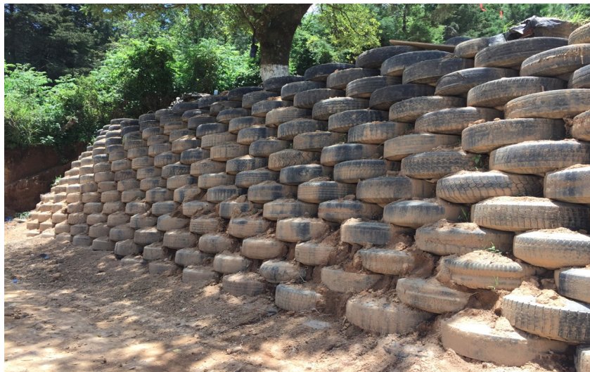
Figure 5.4 - Retaining wall of tires at entrance to LWH campus (Photo: Samantha Hagan)
