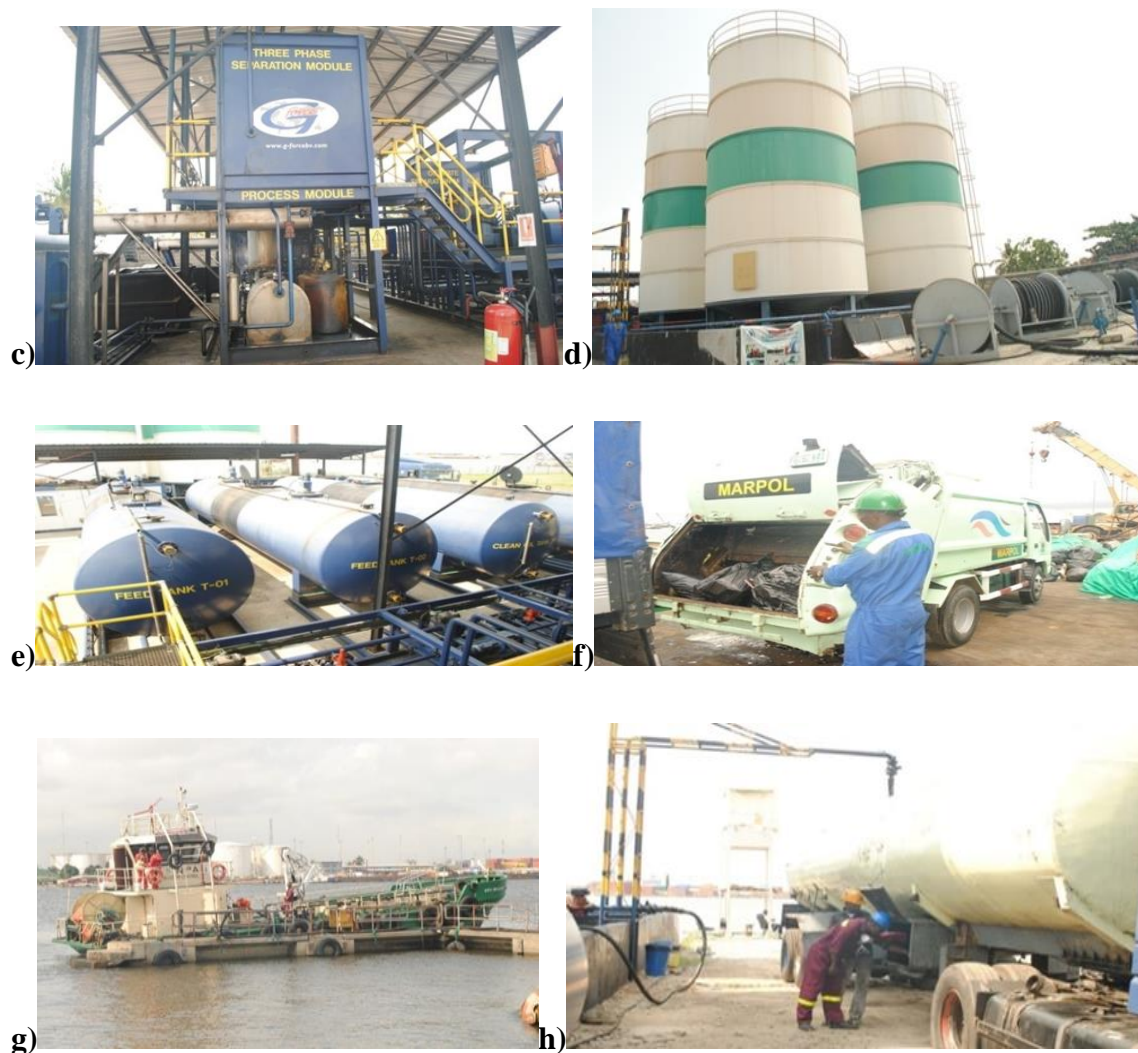
Figure 2 (c to h) Reception facilities use for the implementation of MARPOL 73/78 convention in Nigerian Ports and Terminals
