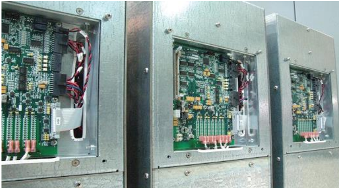
FIGURE III-42: INVERTER MODULE SET
