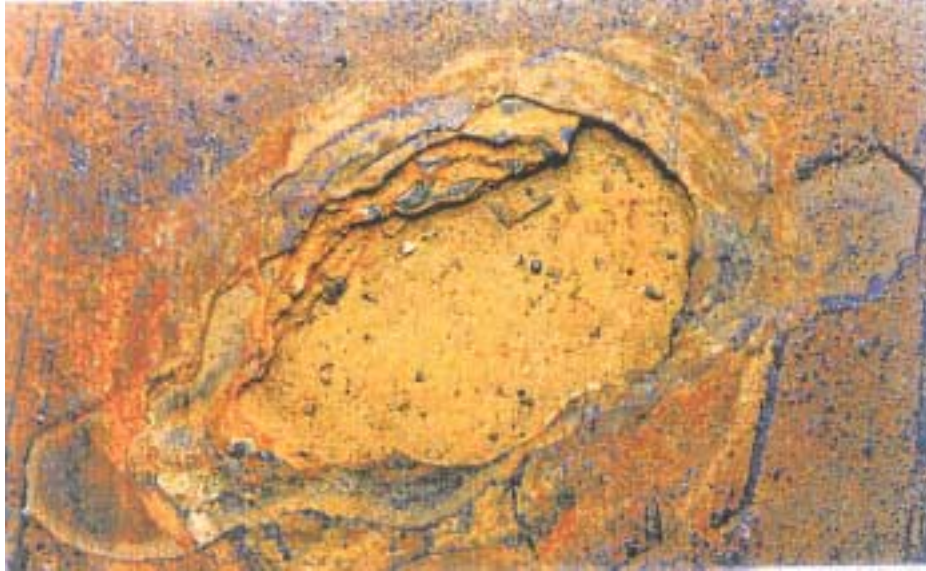
Fig. 21. Pitting corrosion with build up of scale rust in the bottom plate of a ballast tank (Source: DNV paper series No.2000-P008. Appendix 1)
