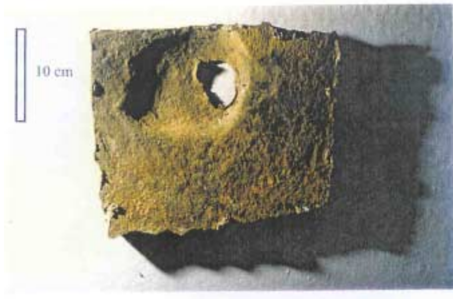
Fig. 19. Severe pitting corrosion in the bottom plate in a combined oil/water ballast tank
