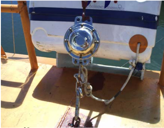
HRU 25 installed upside down.
