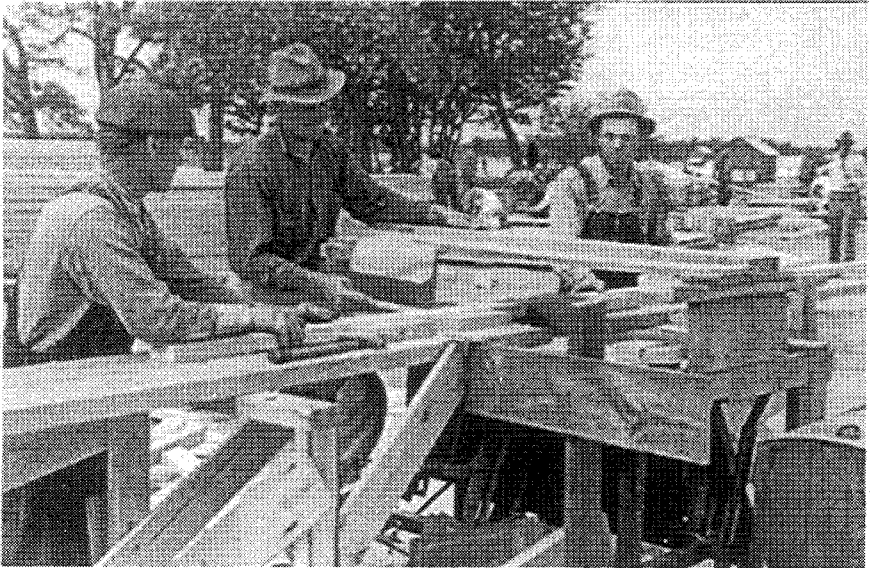
Men construct a prefabricated house at Roanoke Farms Resettlement. Circa late 1930s
