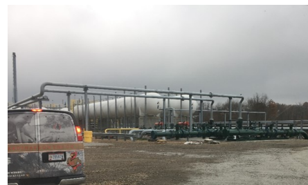
At MarkWest's fractionation facility propane is stored in white tanks pending shipment offsite via rail
