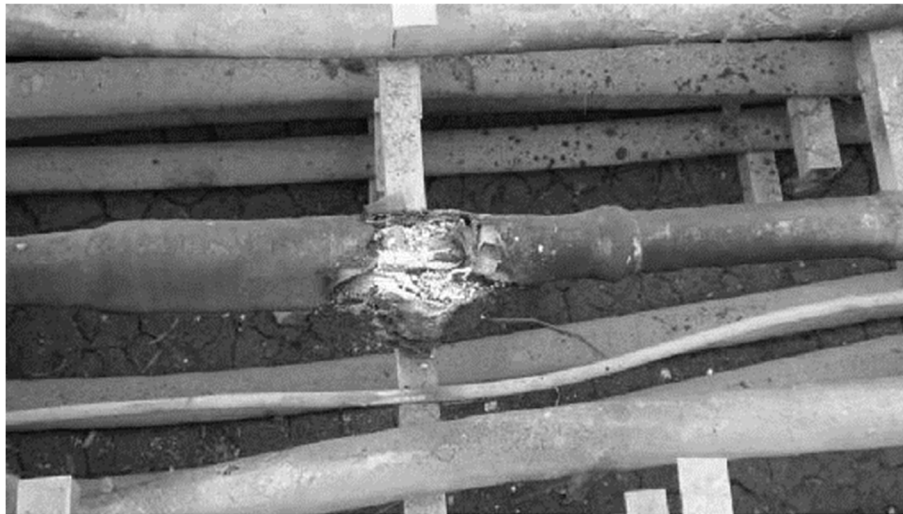
Figure 1-2 Corrupt Cable that Cause Ground Fault
