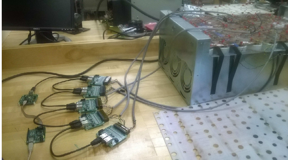
Figure 6.16: 5 BMS boards monitor the Li-ion battery pack voltage and temperature.
