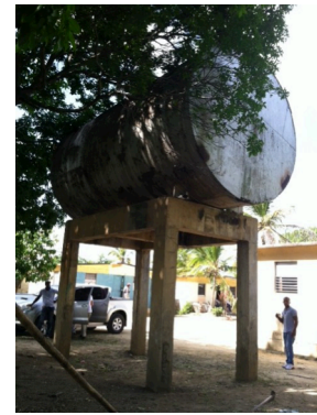
Figure 4: Batey 22 source tank serving Batey 22 and Batey Tentación
