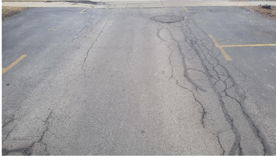
Figure 2.10 Rutting Damage Caused by Traffic Loads
