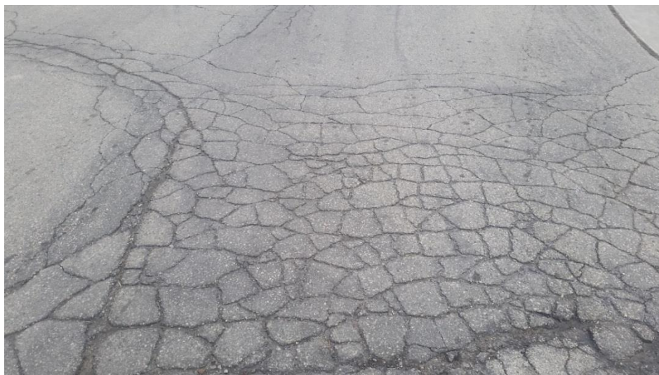
Figure 2.11 Asphalt Fatigue (Alligator) Cracking
