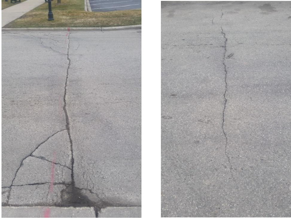
Figure 2.12 Low-Temperature Thermal Cracking
