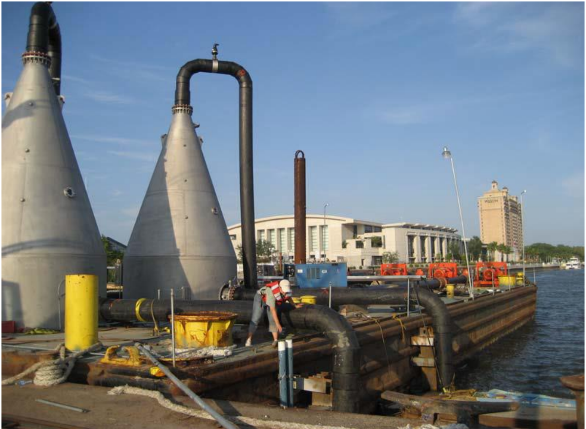
( Figure 2. Savannah Harbor ReOxygenation Demonstration Project. Source: Tetra Tech 2008, p.15)
