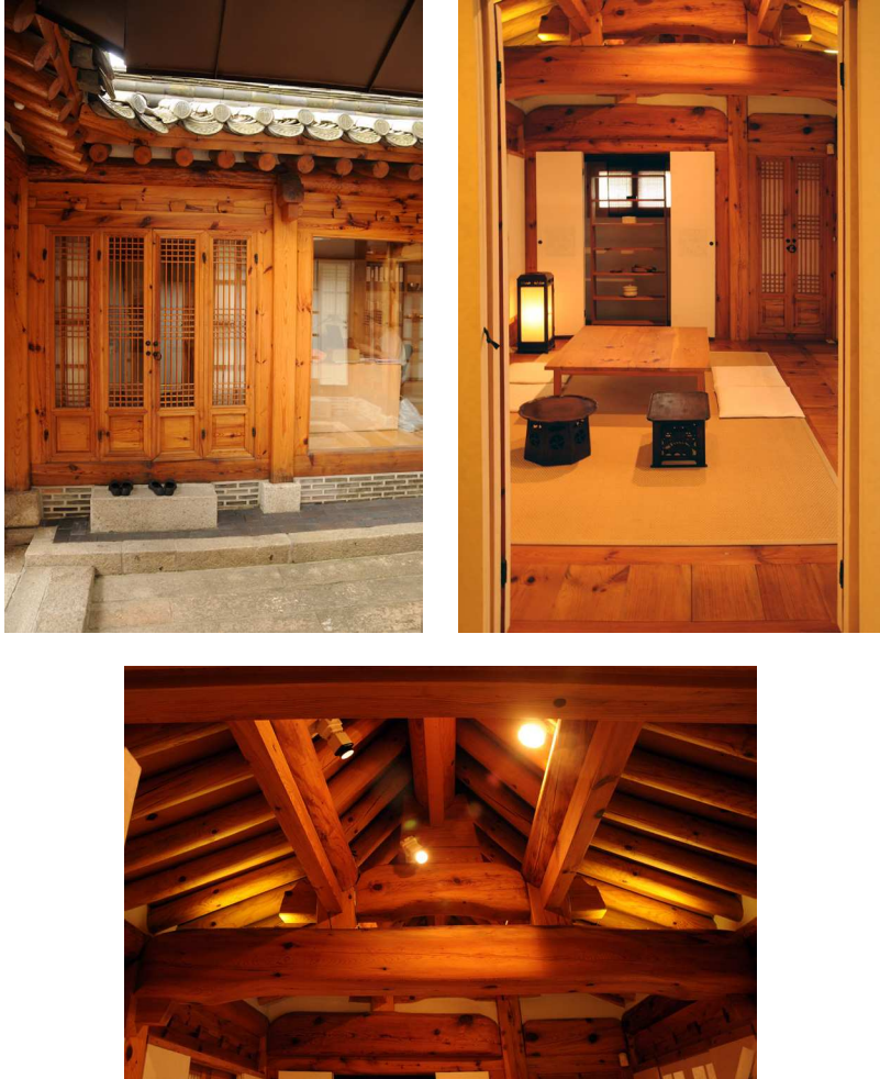
Figure 3. A typical hanok, which consists of a timber frame structure, a unique wood joint system, and a baked tile roof, as frequently shown in popular media. This picture was taken in one of the recent restoration projects in the Bukchon (photo by the author)
