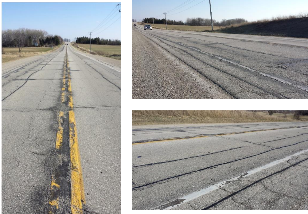
Figure 4.18: Pavement survey distresses observed on a representative 150-ft section on STH 26.
