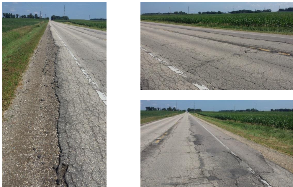
(b) Pictures of various pavement surface distresses
