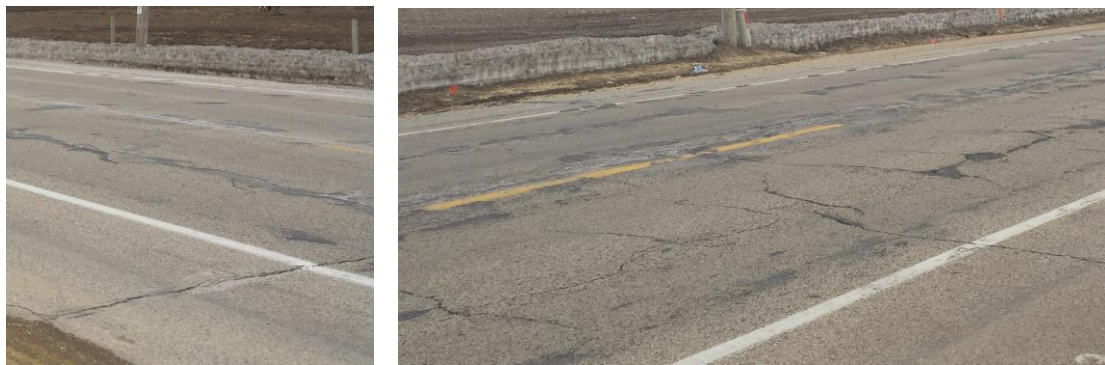
Figure 4.14: Pavement surface distresses observed on STH 11
