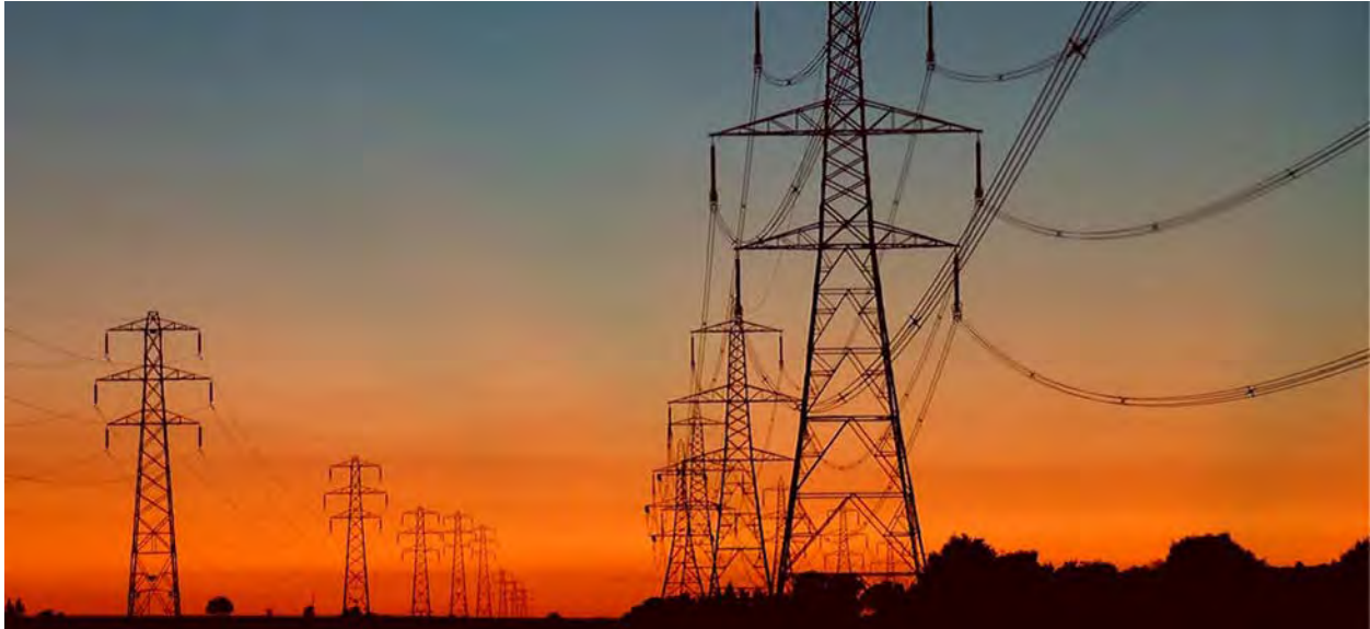
Figure 15.1 The current we draw into our houses is an alternating current (ac). Power lines transmit ac to our neighborhoods, where local power stations and transformers distribute it to our homes. In this chapter, we discuss how a transformer works and how it allows us to transmit power at very high voltages and minimal heating losses across the lines.
