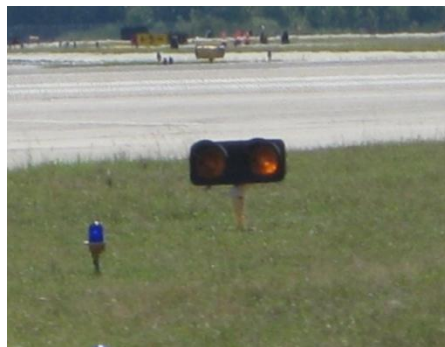
Figure 4. Incandescent Elevated Runway Guard Lights
