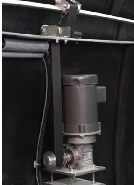
Figure 3.5: The motor and pulley system, located on the inside of the dome.
