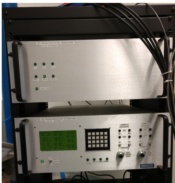
Figure 3.15: The PCS consists of a pneumatics rack (top) and an electronics rack (bottom). The physical user interface is on the bottom rack.
