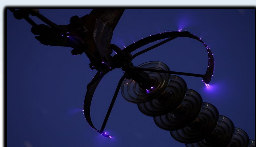
Figure 1: Glow Coronas form on the edges of a powerline transformer (Berkoff, 2005).
