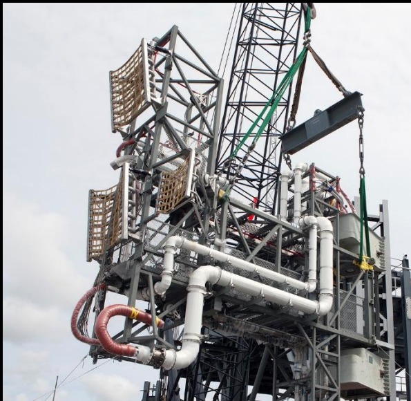
Interim Cryogenic Propulsion Stage Umbilical
