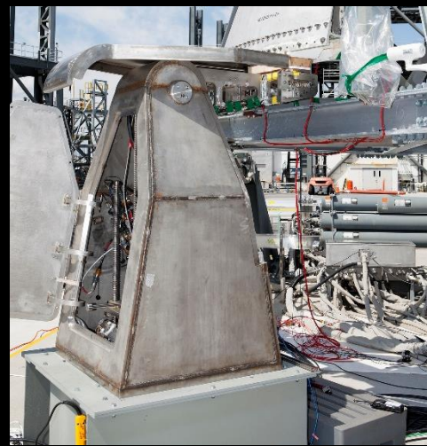
Aft Skirt Electrical Umbilical
