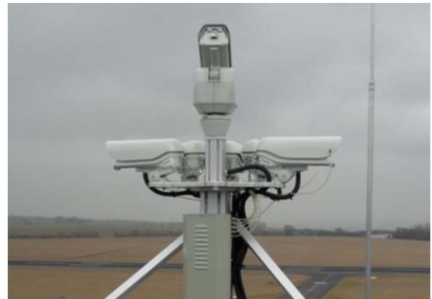
Figure 7. Camera on the top of an airport tower
