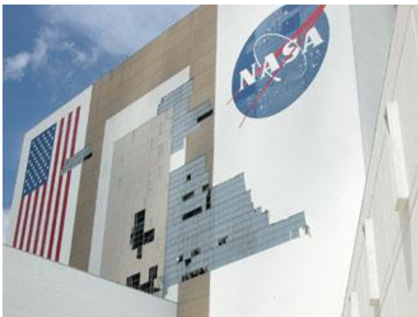
Figure 1. KSC's Vehicle Assembly Building had about 820 panels torn off its south side by Hurricane Frances. Note. Reprinted from NASA's 2004 Hurricane Report.
