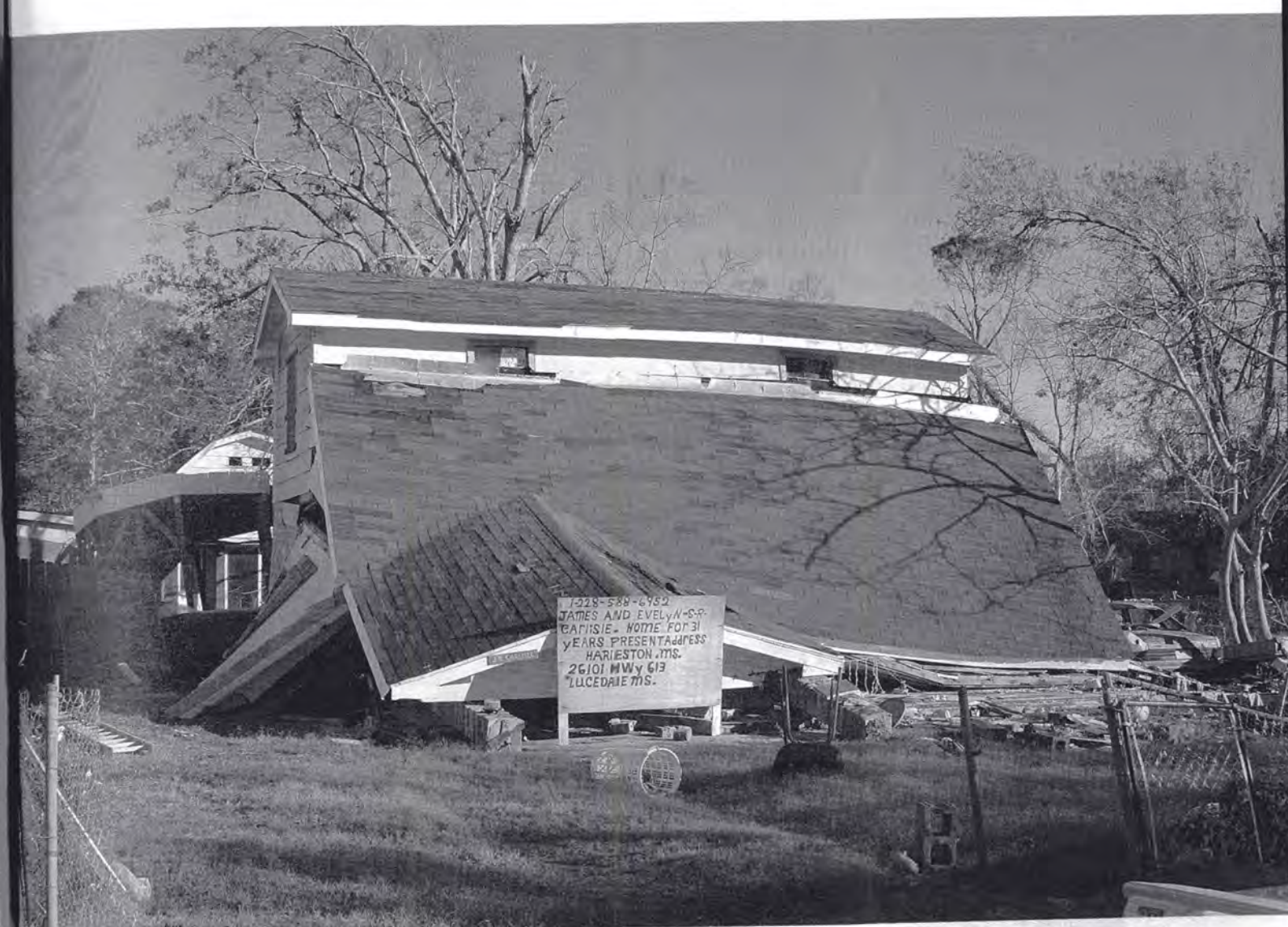
A home in Pascagoula, Mississippi destroyed by Katrina
