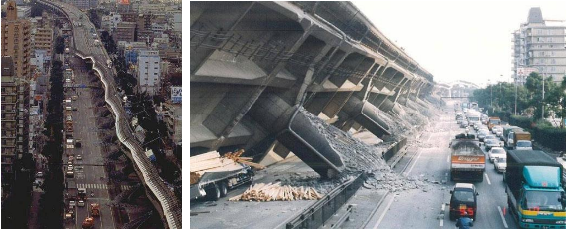
Figure 1.2 Collapsed section of the Hanshin Expressway during the Hyogoken-Nanbu Earthquake (Akai et al., 1995).
