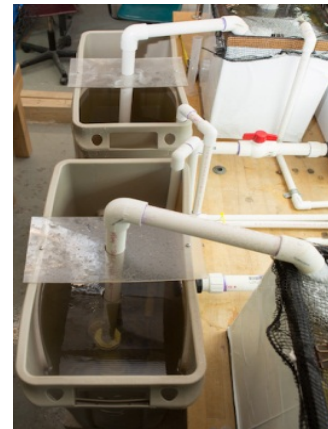
Figure 8: A picture of the airlift piping system. It is located in the sump tank. Top right: the overflow pipe (w/ ball valve) from GB to sump.
