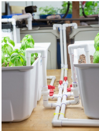
Figure 9: A picture of the valve arrangement. It allows for easy access to adjust the air flow.
