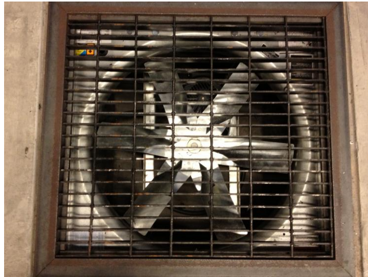
3.21: Intake Fan and Steel Grate
