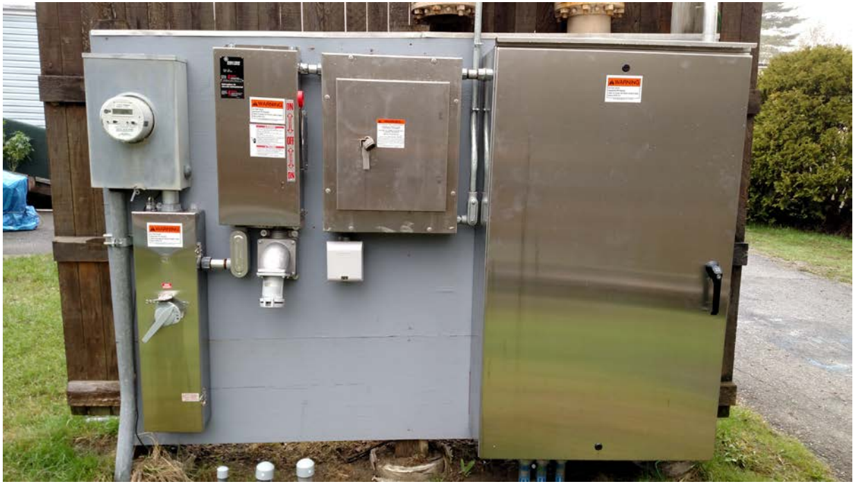
New controls at the Romaha pump station
