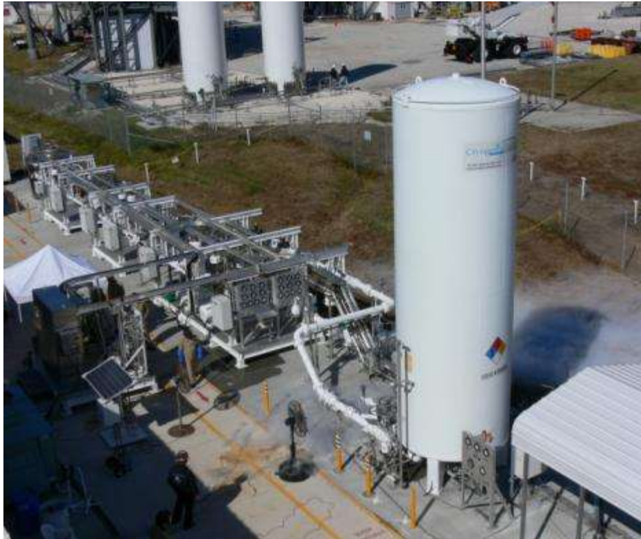
Overall view of the Simulated Propellant Loading System located at the CryoTestLab
