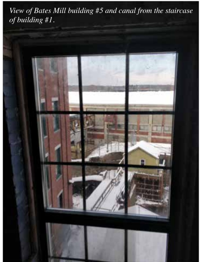
4th and top floor of the Bates Mill with some broken floor boards. There are no occupants in this room, and is currently under renovation.
