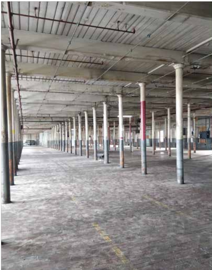
Floor 3 of the Bates Mill. There are no occupants in this room, it is under renovation.
